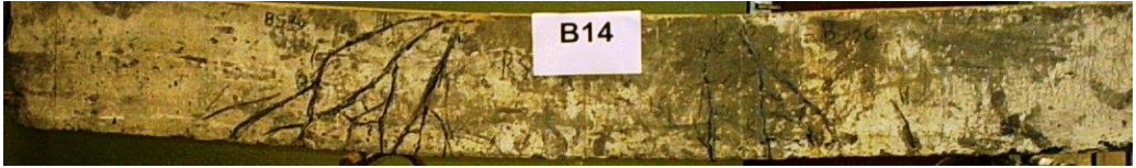
Fig. 2.h: Pattern of crack of the tested beam (B14).
