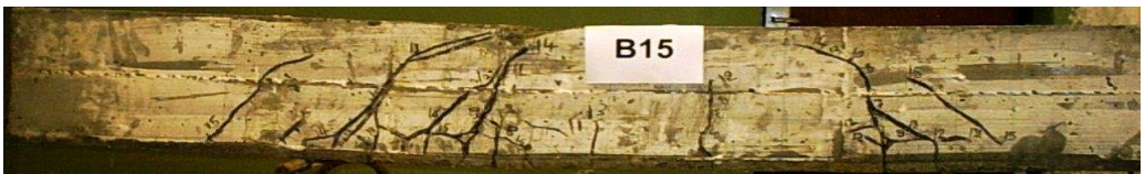
Fig. 2.i: Pattern of crack of the tested beam (B15).
