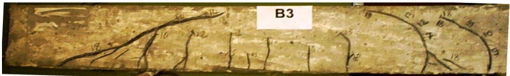
Fig. 2.c: Pattern of crack of the tested beam (B3).
