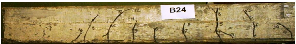
Fig. 2.m: Pattern of crack of the tested beam (B24).
