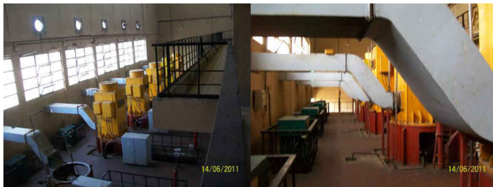
a) Motors inside the pumping station building
