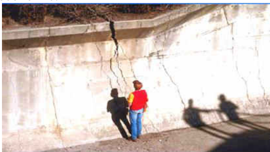
Photo 2. Wall Failure along Dam Spillway (Mark G. Thomas 2008)
