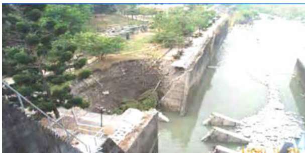
Photo 1. Some Problems due to expansive soils (Mark G. Thomas 2008)
