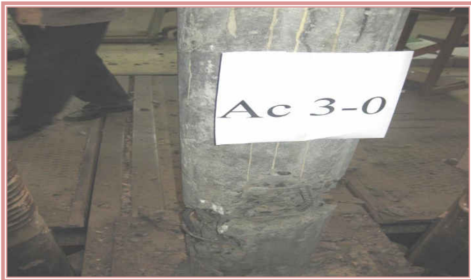
Failure mode, the first mechanism, (Ac 1-0), (Ac 2-0) and (Ac 3-0) (unconfined circular R.C. columns)( FM 1)
