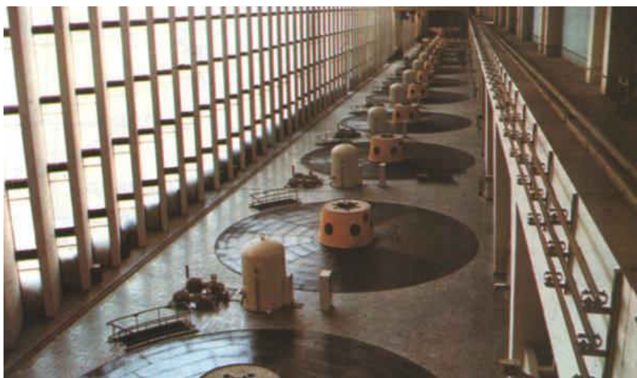
Fig. 5. Photographic view inside the power house.
