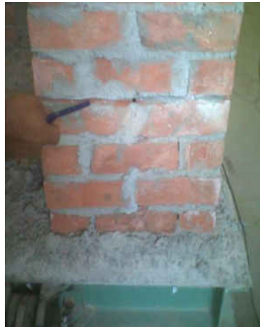
Fig. 7. Artificial crack formation.
