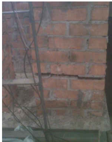
Fig. 6. Crack location determination test.
