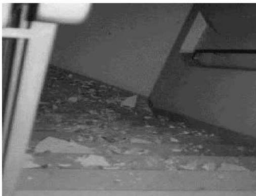
Fig. 37. Emergency staircase blocked with garbage
