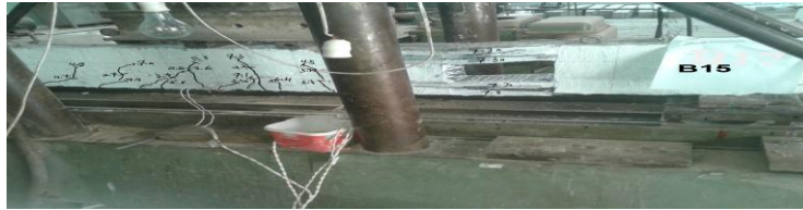
Photo 18. Crack pattern of beam "B15".
