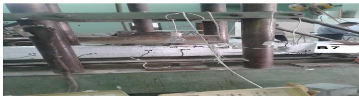
Photo 10. Crack pattern of beam "B7".
