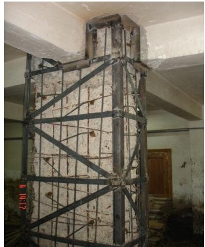
Plate (2) The steel angles and both the transverse and diagonal plates of the jacket.
