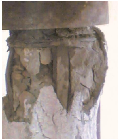
Figure (16) Buckling of the vertical steel plates of the circular column.
