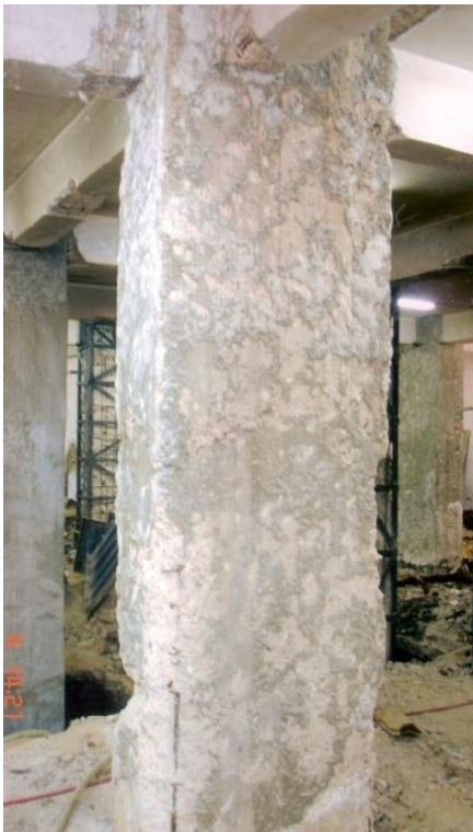
Plate (1) Deteriorated column before applying the steel jacket.
