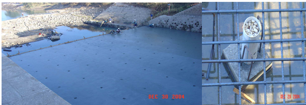
Fig. (2): The final surface of apron with relief wells (left side) – R.w pipe filled with gravel
