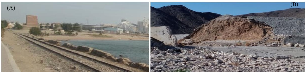
Figure 20 Examples of ineffective implemented treatment methods: (A) Failure of Stone-built barriers, (B) Embankment failure.
