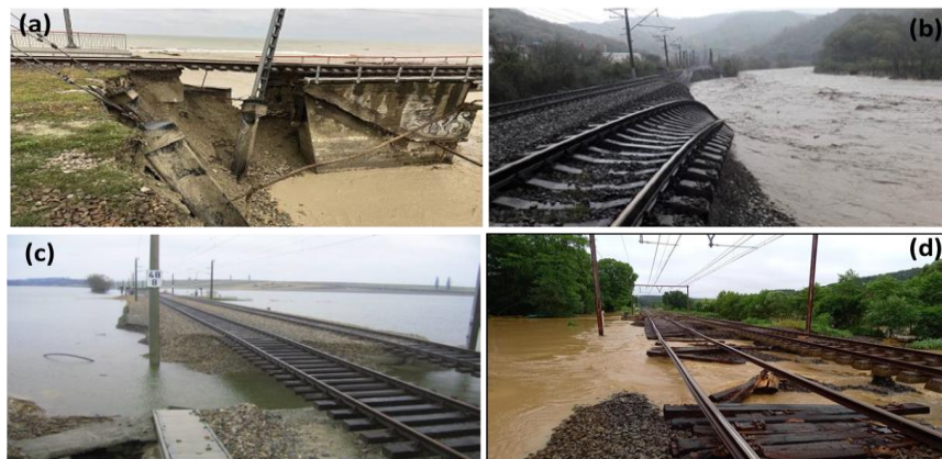
Figure 6 Some cases of flood damage, (a) Railway bridge scour; (b) Railway infrastructure damage in Russia [6]; (c) Rail damage in Austria [2]; and (d) Rail damage in Belgium [7].
