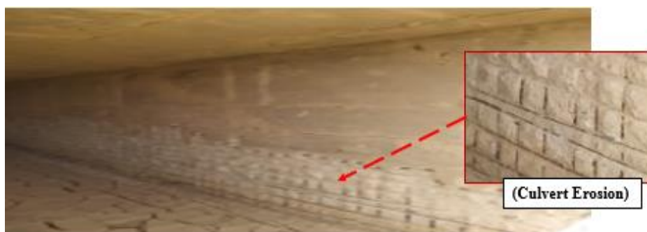
Figure 19 Flood erosion for a sediment-filled culvert wall (Egyptian Railways).
